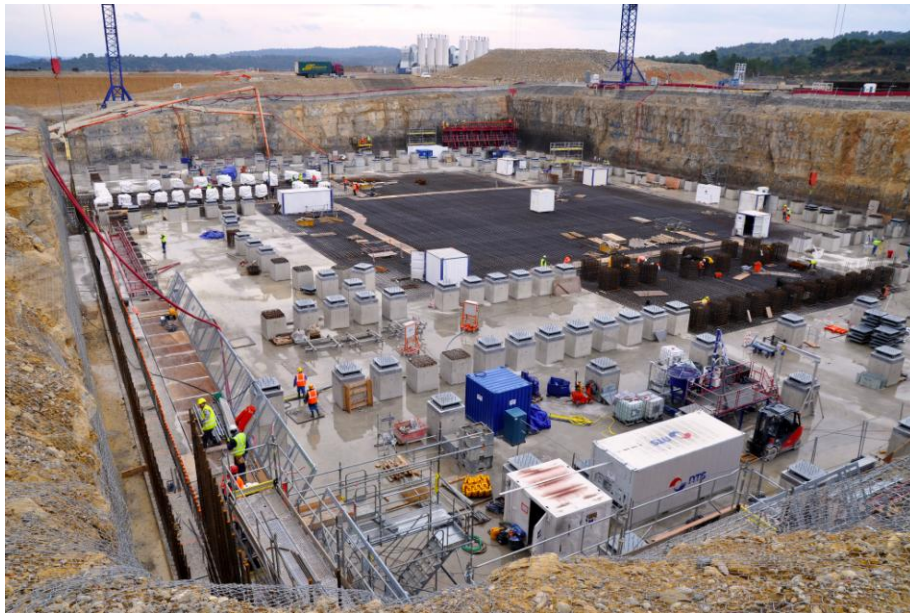
Seismic pads, all in a row
